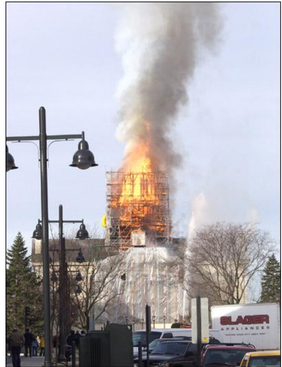
Figure 12: The Old Cap fire caused by an out-of-state, low-wage contractor using cheaper but prohibited heat techniques to remove paint and asbestos
